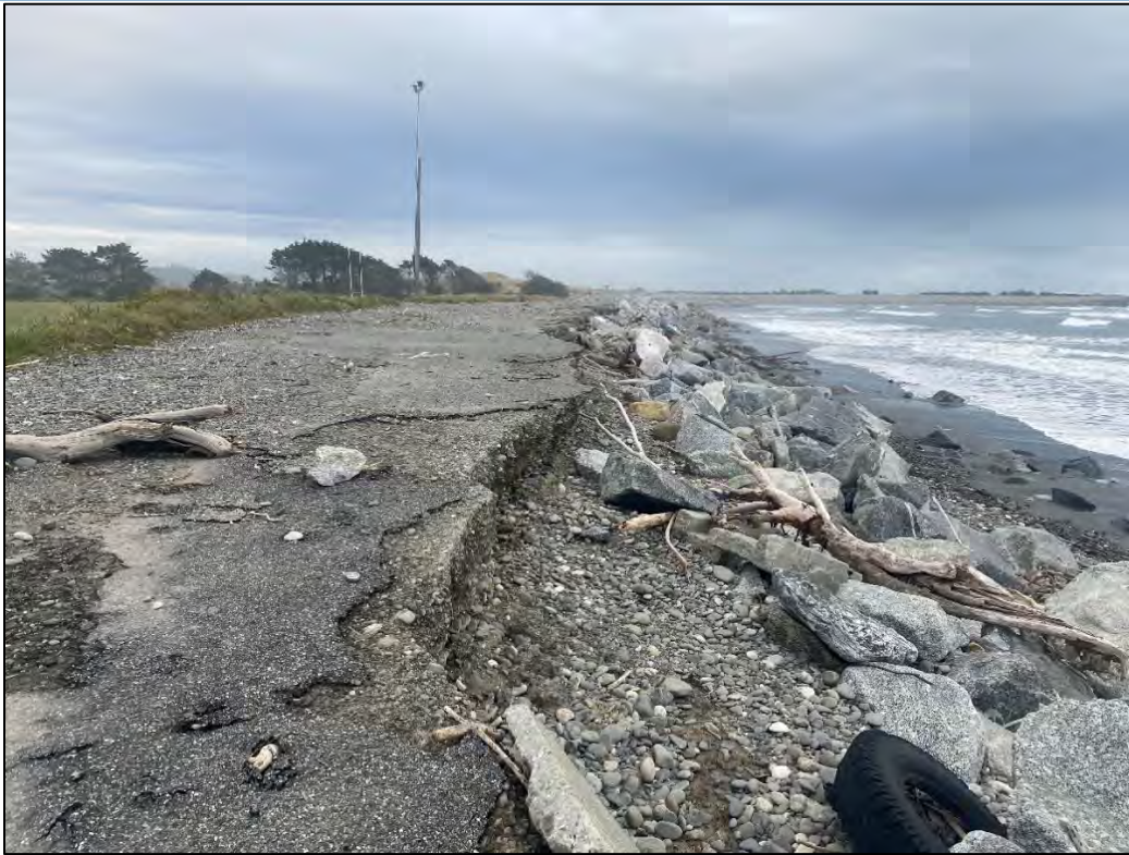
Figure 2-2 – Mid section of wall, collapsing and in serious need of repair (adjacent to Jellyman park)
