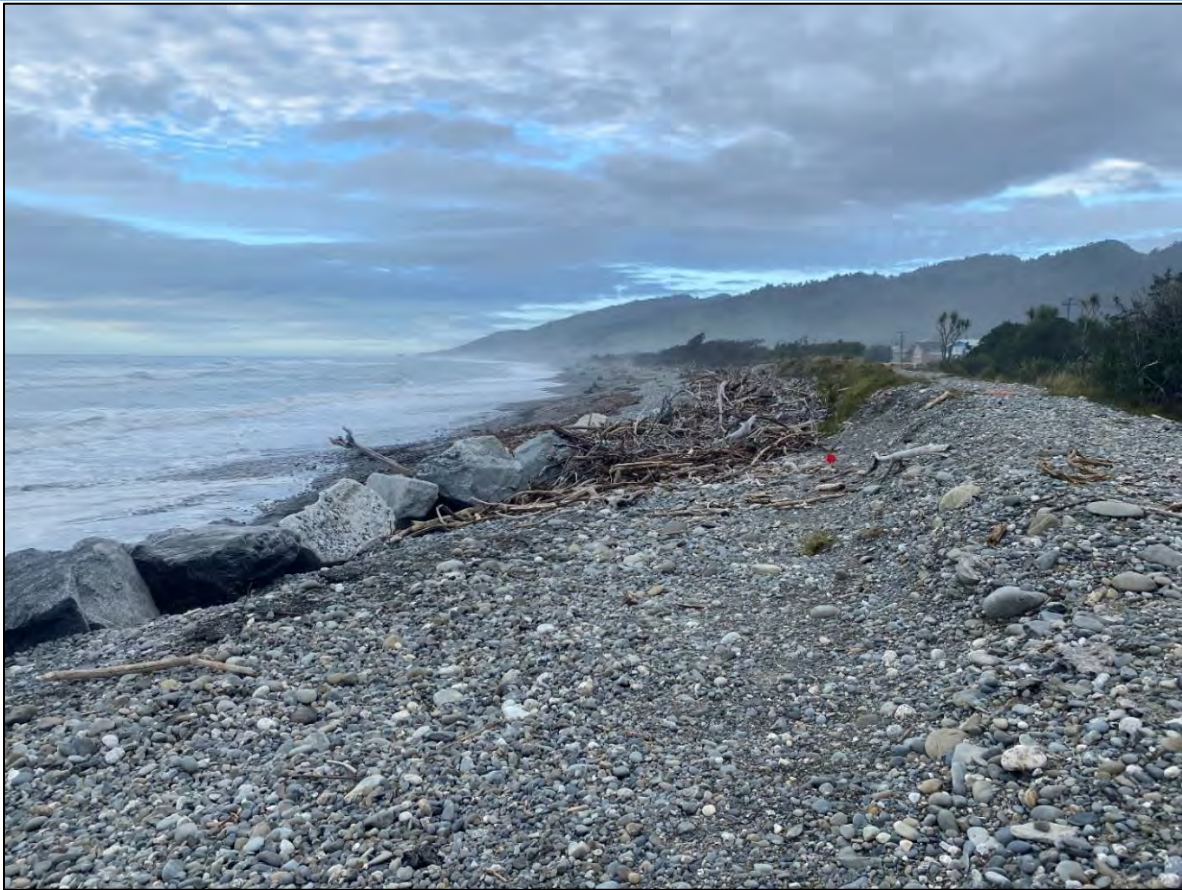
Figure 2-5 – Northern most section of the wall with no current rock protection
