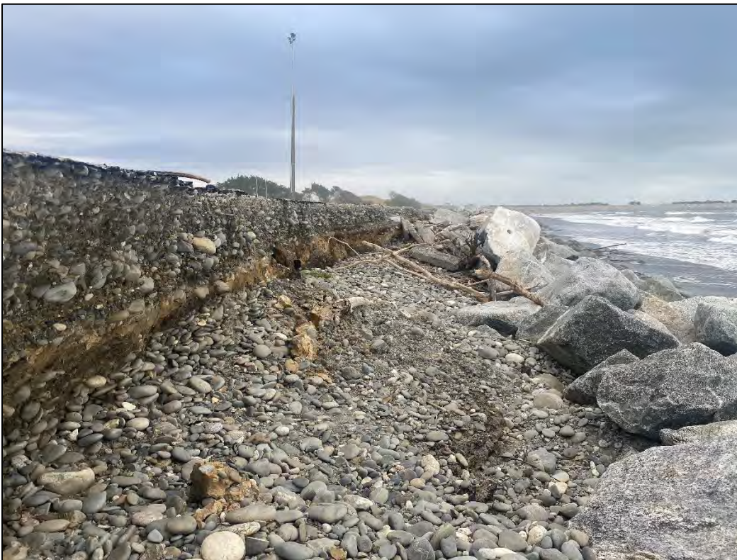
Figure 2-3 – Severe erosion of the wall
