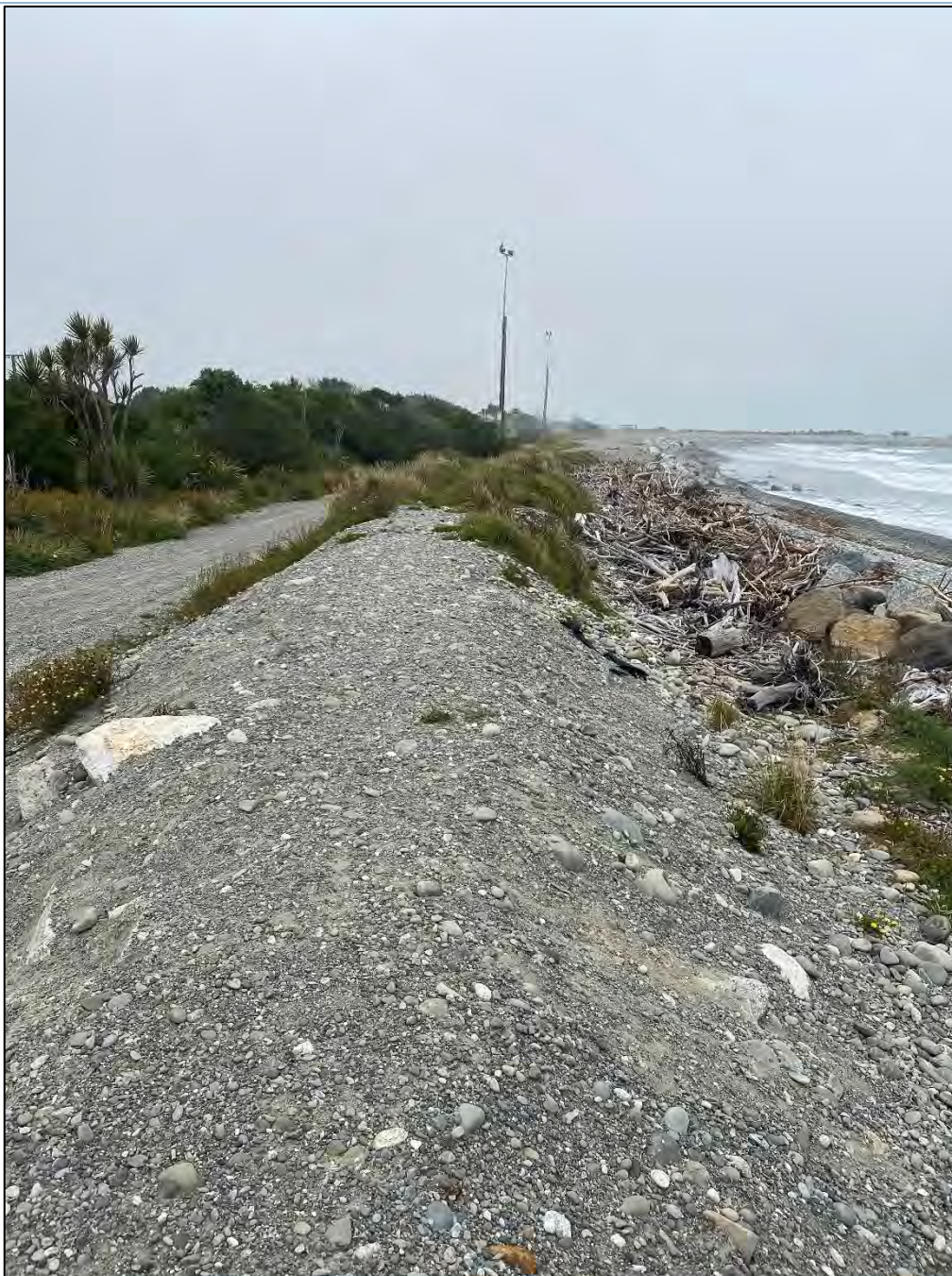
Figure 2-6 – Gravel bund easily erodible by the sea during a storm event
